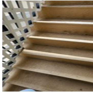
Picture 30 ( Defect Code: 59 ) Link (click to view High-Res)
