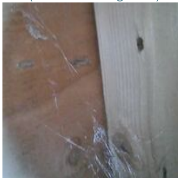
Picture 368 ( Defect Code: 240 ) Link (click to view High-Res)
