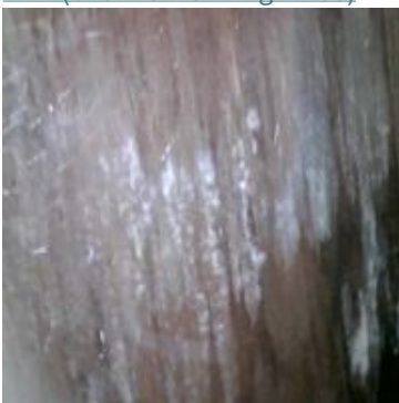
Picture 361 ( Defect Code: 137 )
