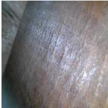
Picture 365 ( Defect Code: 202 ) Link (click to view High-Res)
