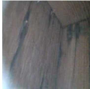
Picture 366 ( Defect Code: 202 ) Link (click to view High-Res)
