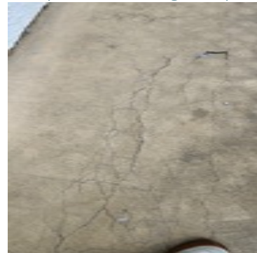
Picture 177 ( Defect Code: 19 )
