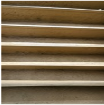
Picture 29 ( Defect Code: 59 ) Link (click to view High-Res)
