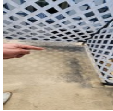
Picture 183 ( Defect Code: 35 )
