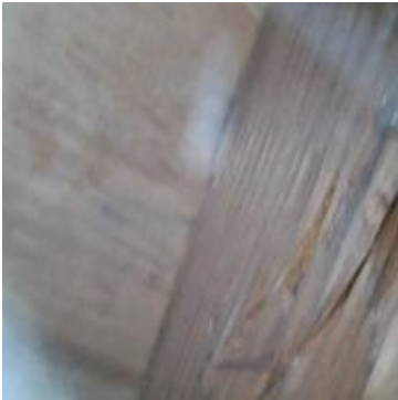
Picture 364 ( Defect Code: 202 ) Link (click to view High-Res)
