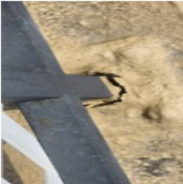
Picture 243 ( Defect Code: 122 ) Link (click to view High-Res)
