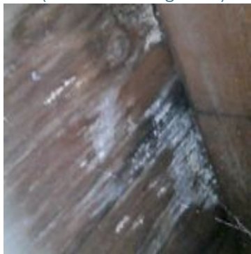
Picture 359 ( Defect Code: 137 )
