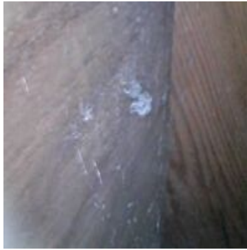
Picture 98 (Defect Code: 147)
