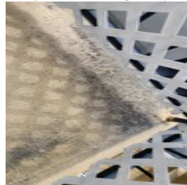
Picture 186 ( Defect Code: 61 )
