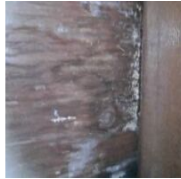
Picture 357 ( Defect Code: 137 )
