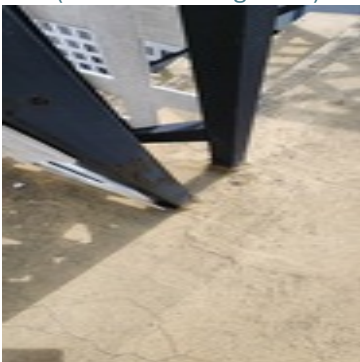
Picture 255 ( Defect Code: 101 ) Link (click to view High-Res)
