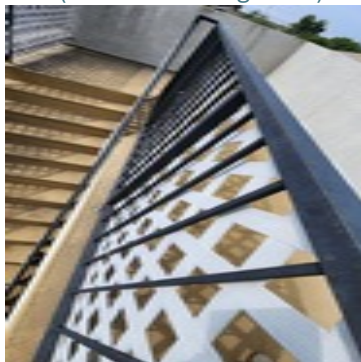
Picture 247 ( Defect Code: 109 ) Link (click to view High-Res)
