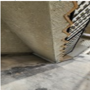
Picture 69 ( Defect Code: 133 )
