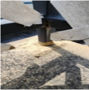
Picture 252 ( Defect Code: 101 ) Link (click to view High-Res)
