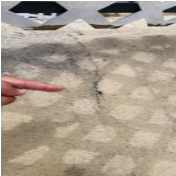
Picture 175 ( Defect Code: 19 )
