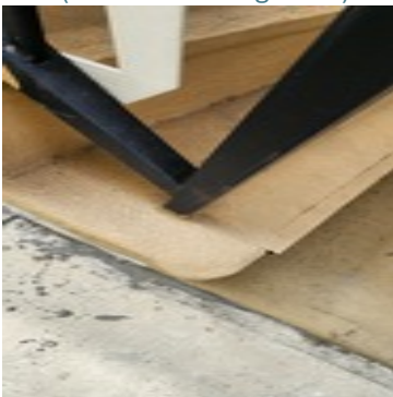
Picture 61 ( Defect Code: 100 )
