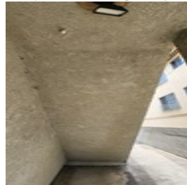
Picture 68 ( Defect Code: 133 )
