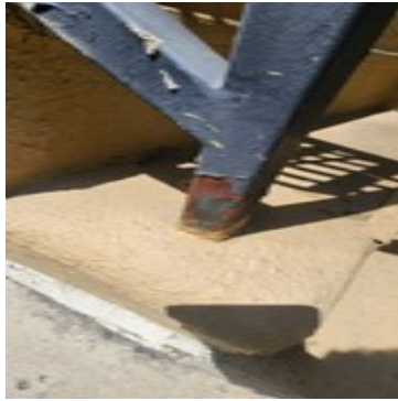
Picture 437 (Defect Code: 101)
