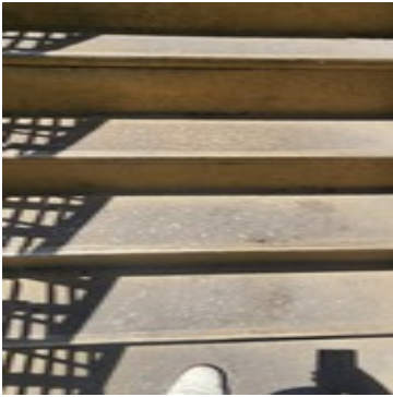
Picture 407 ( Defect Code: 59 ) Link (click to view High-Res)
