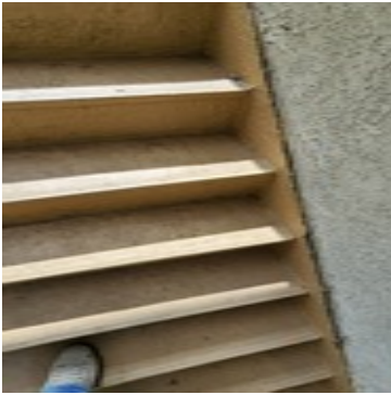
Picture 28 ( Defect Code: 59 ) Link (click to view High-Res)
