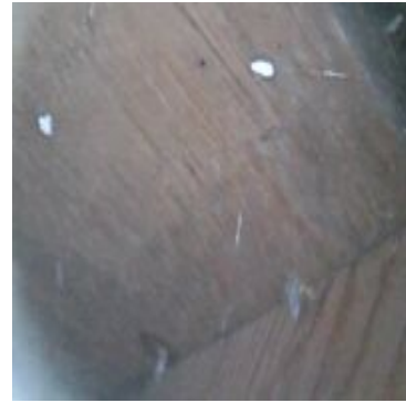
Picture 99 (Defect Code: 147)
