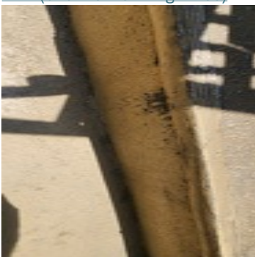
Picture 404 (Defect Code: 17)
