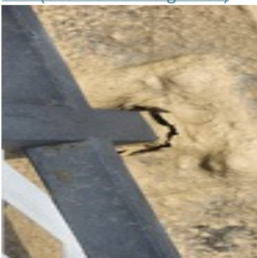
Picture 249 ( Defect Code: 113 ) Link (click to view High-Res)
