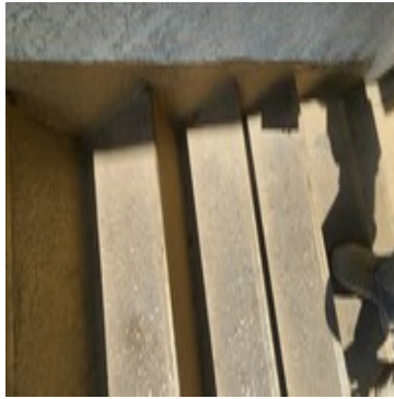
Picture 408 ( Defect Code: 59 ) Link (click to view High-Res)
