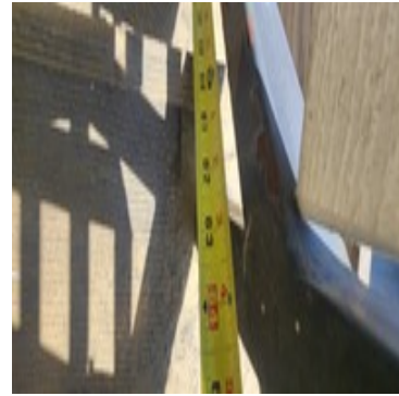
Picture 438 (Defect Code: 101)
