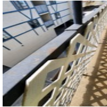
Picture 254 ( Defect Code: 101 ) Link (click to view High-Res)
