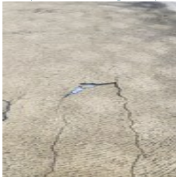
Picture 176 ( Defect Code: 19 )
