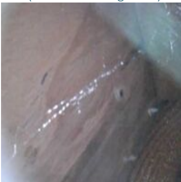
Picture 367 ( Defect Code: 240 ) Link (click to view High-Res)
