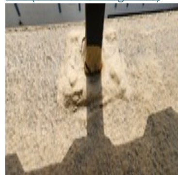
Picture 251 ( Defect Code: 101 ) Link (click to view High-Res)
