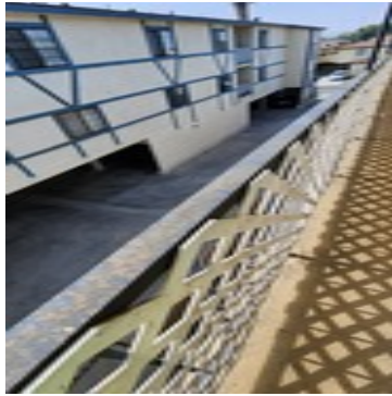
Picture 253 ( Defect Code: 101 ) Link (click to view High-Res)
